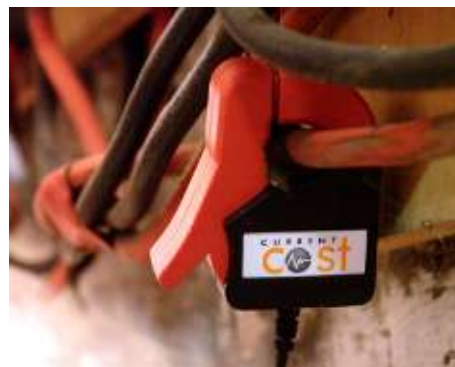
Figure 2.1.: The Current Cost clamp installed in our home.
